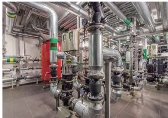
Municipal heating system
